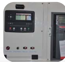
Control Panel & MCB
